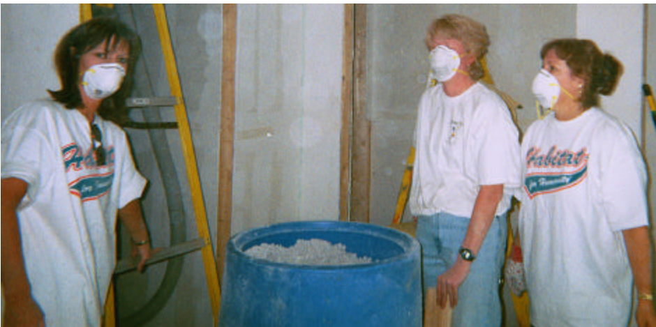
. . . Mary Regan, Jodi Stanislawski and Deb Bowser keep the hopper full of insulation
